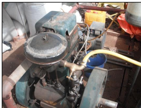
Figure 20: Tap connection for biogas supply
